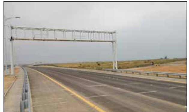
Four lanes of traffic on each approach have Intercomp WIM Strip Sensors installed.
