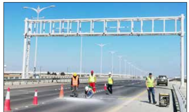
WIM sensors are installed in the existing roadway and ground flush with the pavement surface.
