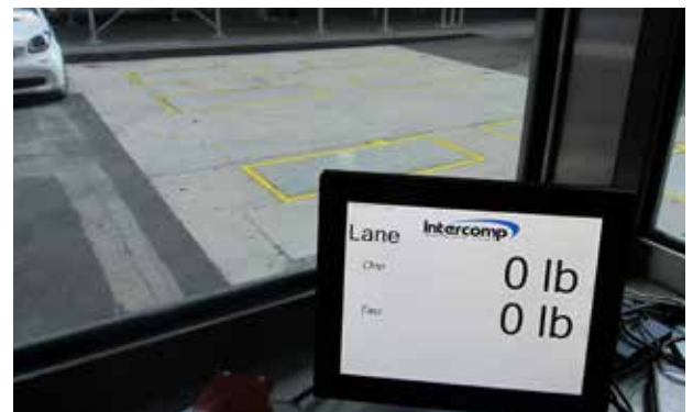
Each lane reports vehicle weights for security personnel to monitor for dangerous goods.
